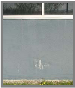
Efflorescence on finish coat
