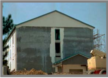
Efflorescence on base coat
