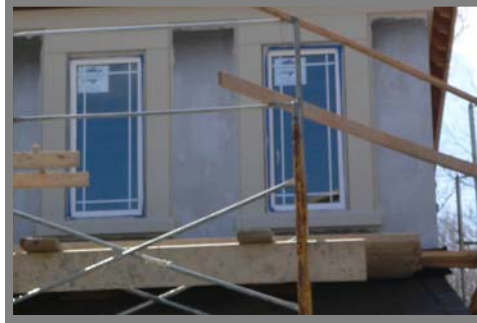
Efflorescence on base coat
