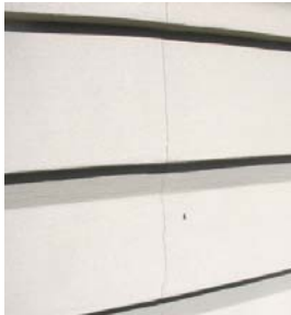
Cracked joint in EIFS trim
